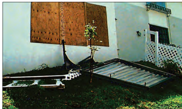
Figure 3. Hurricane Georges in Puerto Rico. The window lying on the ground was protected by a shutter. However, the shutter was attached to the window frame. The window frame fasteners were over-stressed and the entire assembly failed. Attachment of the shutter directly to the wall framing is a more reliable method of attachment.
