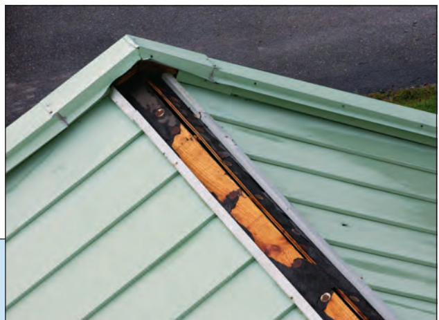
Figure 9. The ridge flashing fasteners were placed too far apart. A significant amount of water leakage can occur when ridge flashings are blown away.
