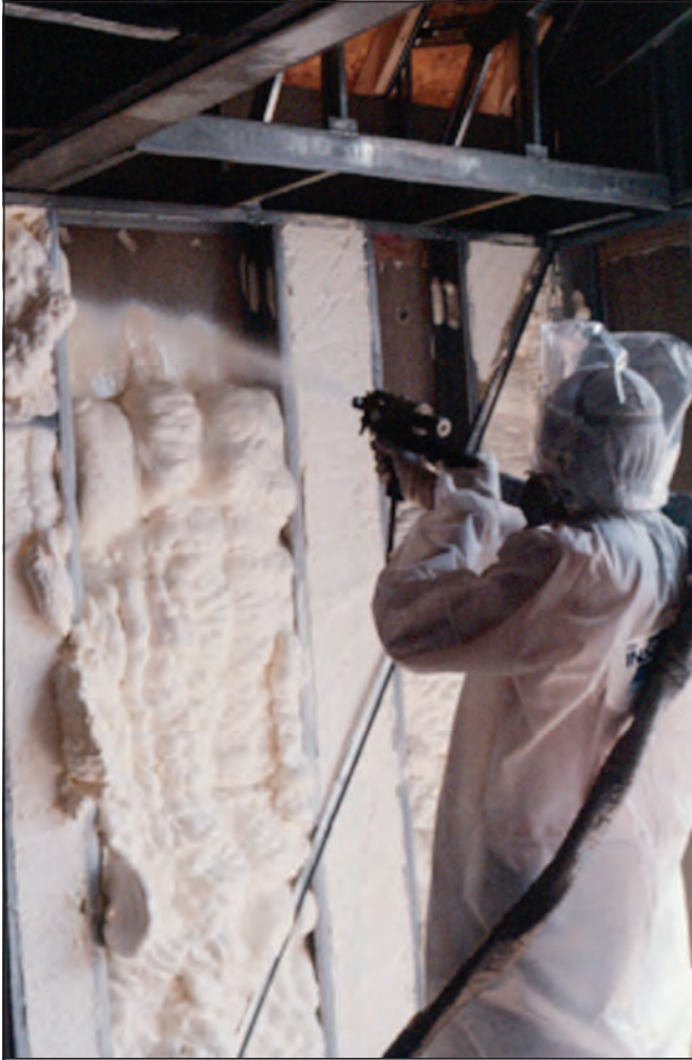
Figure 5. An example of a wall cavity filled with sprayed closed-cell foam insulation.
