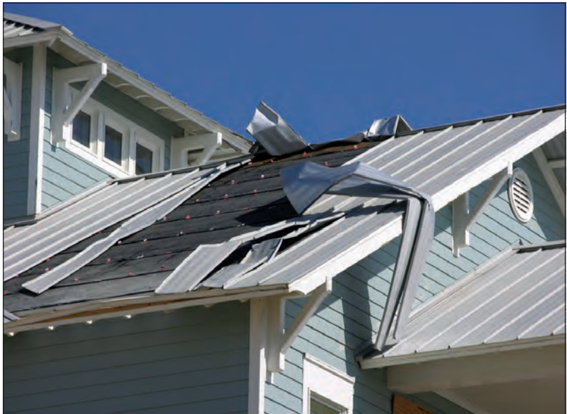
Figure 2. This architectural panel system has concealed clips. The panels unlatched from the clips. The first row of clips (just above the red line) was several inches from the end of the panels. The first row of clips should have been closer to the eave.
