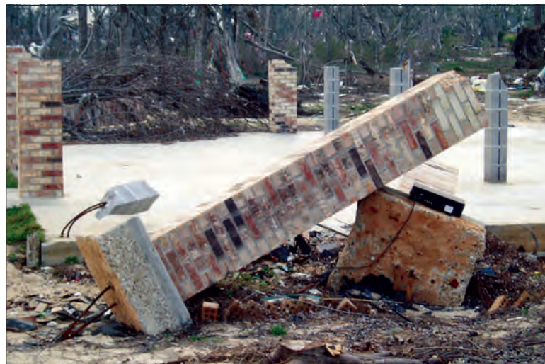
Figure 2. Performance comparison of pier foundations. Piers on discrete footings (foreground) failed by rotating and overturning while piers on more substantial footings (in this case a concrete mat) survived (Pass Christian, Mississippi)
