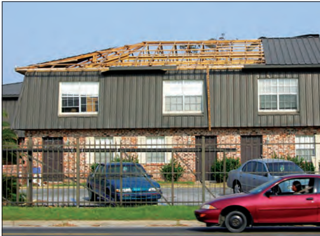
Figure 6. Blow-off of nailers caused these panels to progressively fail. The nailers were installed directly over the trusses. In an assembly such as this where there is no decking, there is no opportunity to incorporate an underlayment. With loss of the panels, rainwater was free to enter the building.
