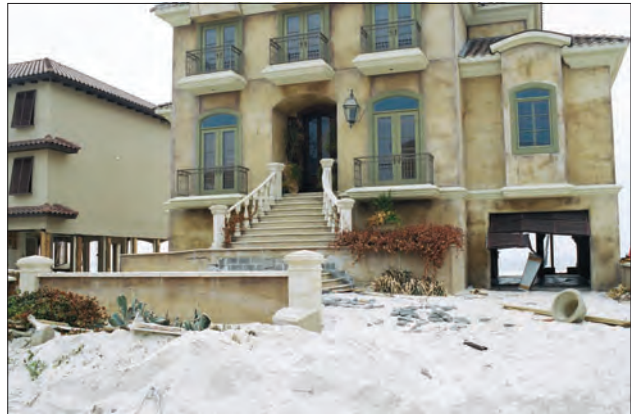
Large solid stairs such as these block flow under a building and are a violation of NFIP free-of-obstruction requirements.
