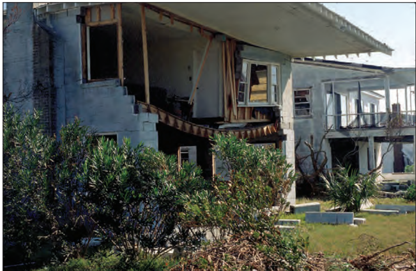
Figure 1. Storm-damaged homes need repairs, but also provide opportunities for renovation, additions, and retrofitting. Review substantial damage and substantial improvement regulations before undertaking any work.
