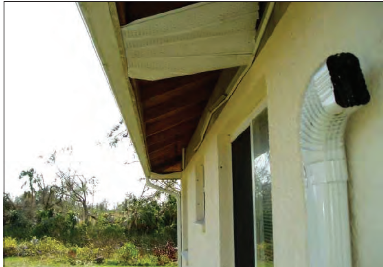
Figure 1. Missing soffit material.
