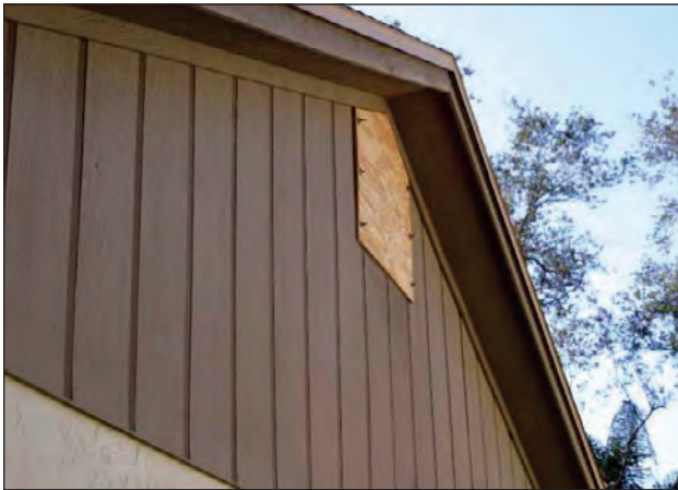
Figure 10. Shuttered gable end vent.
