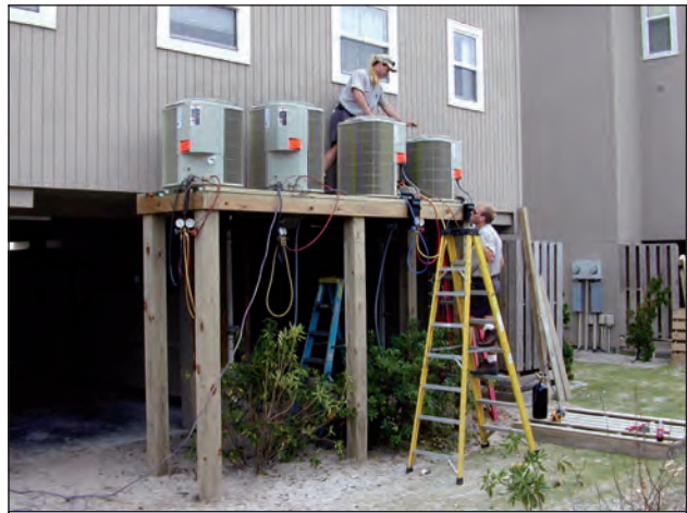
Elevated air conditioning compressors.
