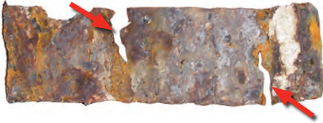
Figure 3. Significant tie corrosion caused the brick at a fire station to fail, even though the building is not near the coast. Note that metal is missing for half of the width of the tie at two locations (red arrows). The left end of the tie was still embedded into a concrete masonry unit back-up wall. The right end is where the tie failed in tension, thus leaving a portion of the tie embedded in the collapsed brick.
