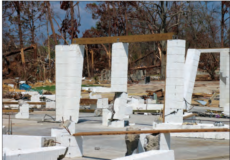
Figure 2. Pier breakage (Long Beach, Mississippi)
