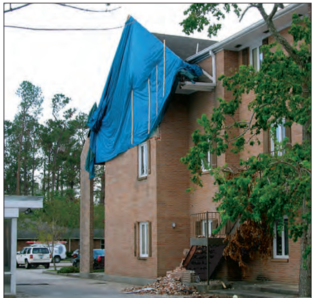
Figure 2. The upper portion of the brick veneer at this apartment building collapsed. Pedestrian and vehicular traffic in the vicinity of the damaged wall are vulnerable to injury and damage if remaining portions of the wall were to collapse during subsequent storms.
