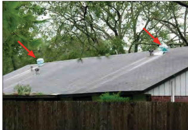
Figure 14. Plastic wrapped turbines.
