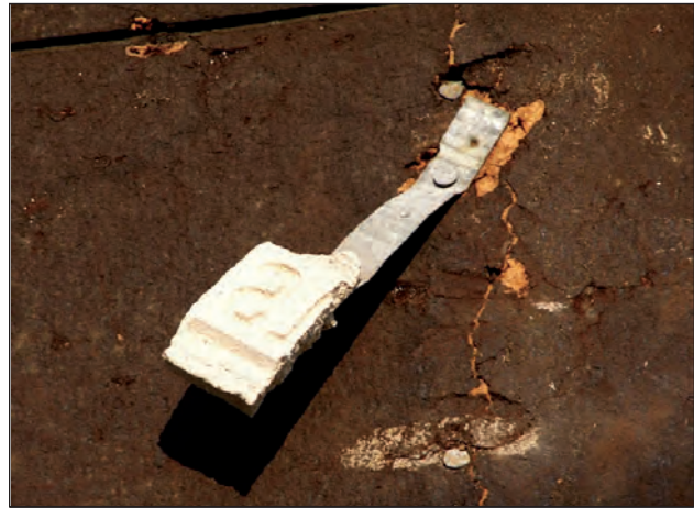
Figure 6. This tie was embedded in the mortar, but the bond was poor.
