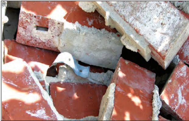
Figure 4. This tie remained embedded in the mortar joint while the smooth-shank nail pulled out from the stud.
