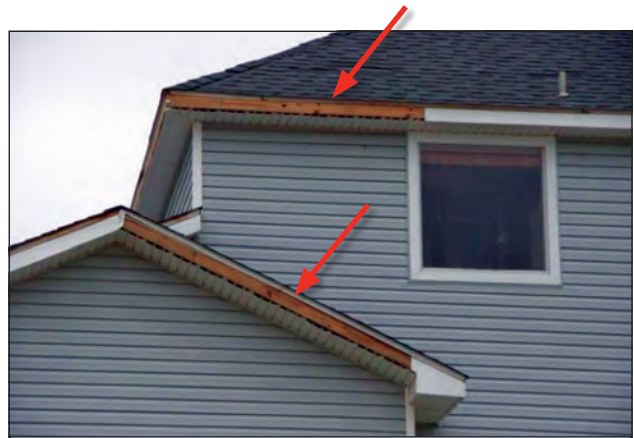
Figure 7. Loss of fascia cover exposes ends of vinyl soffit to direct entry of wind-driven rain.
