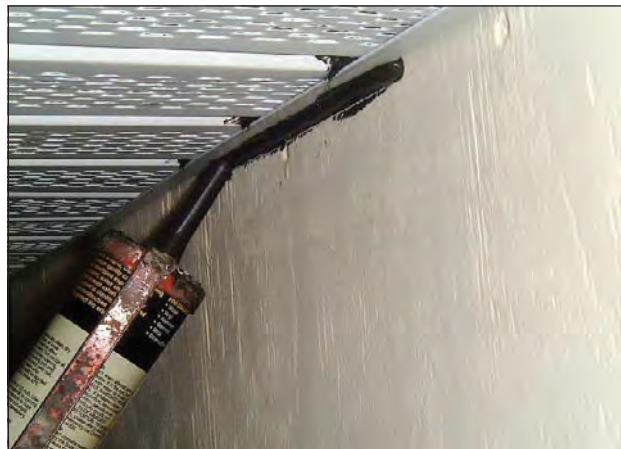
Figure 3. Applying a bead of sealant. (Note: Black sealant was used so that it would be visible in the photograph. Normally a matching sealant color would be used.)
