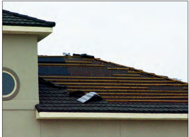
Figure 7. This residence had metal shingles that simulated the appearance of tile. The shingles typically blew off the battens, but some of the battens were also blown away.
