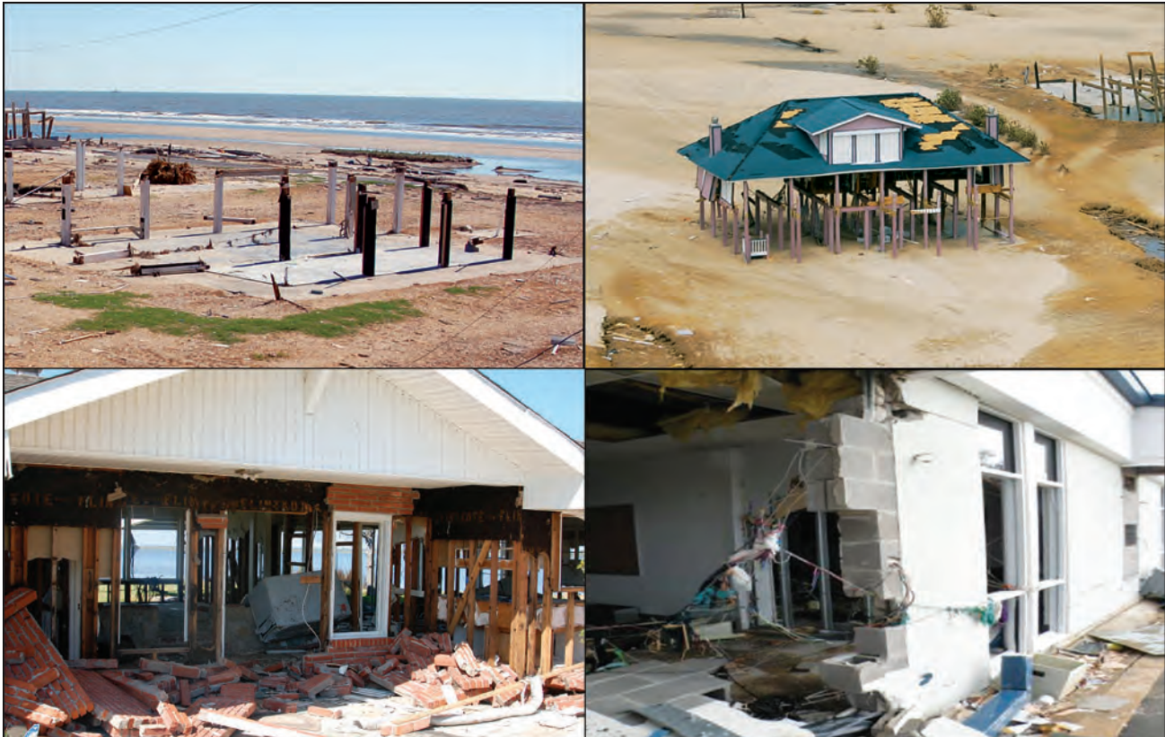
Figure 5. Hurricane Ike damage to buildings. The upper left and upper right photos are of buildings that were close to the Gulf of Mexico shoreline and subjected to storm surge and large waves above the lowest floor. The lower left photo is of a building close to Galveston Bay shoreline and subjected to storm surge and small waves. The lower right photo is of a Cameron Parish, Louisiana, school that was approximately 1.3 miles from the Gulf shoreline, but subjected to storm surge and small waves.
