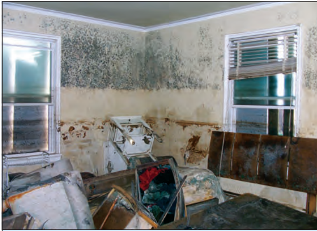
Figure 6. Mold and biological/chemical contamination are also concerns when flood levels rise above the lowest floor. Contamination may result in the building being irreparable or, at least, make the cleanup, restoration, and repairs more expensive and time-consuming.
