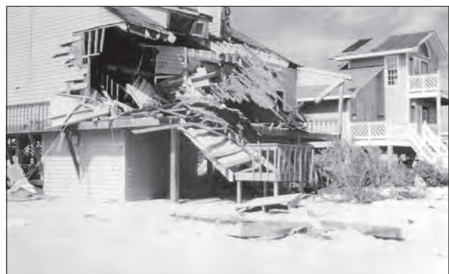
Figure 2. Well-sited building that still sustained damage.
