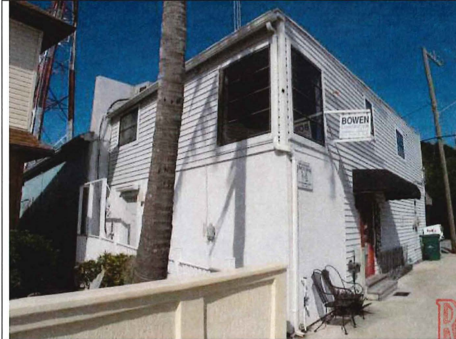
2006 photo from the Property Appraiser’s website shows the side elevation along Palm Ave and the rear (south) elevation as these were. The photo shows the building with a variety of contemporary window types and no historic windows.
