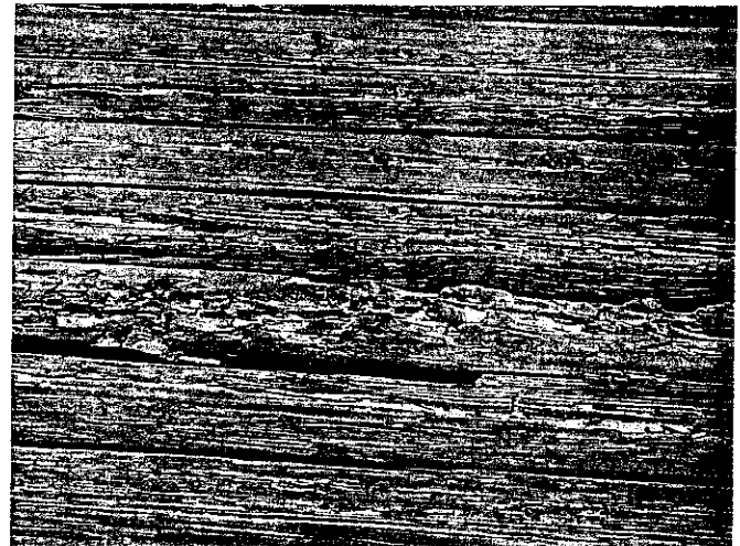
Severe deck deterioration
