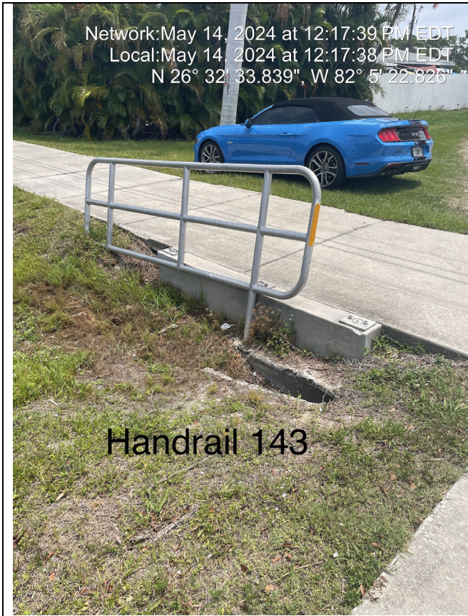
Handrail 143 Post Hurricane
