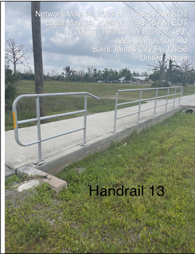
Handrail 13 Post Hurricane
