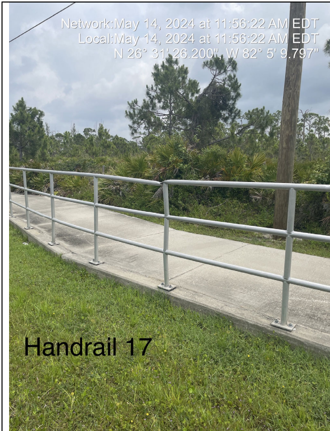
Handrail 17 Post Hurricane
