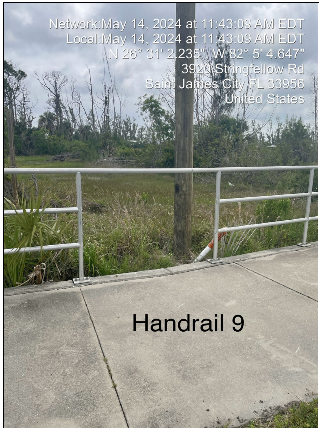
Handrail 9 Post Hurricane
