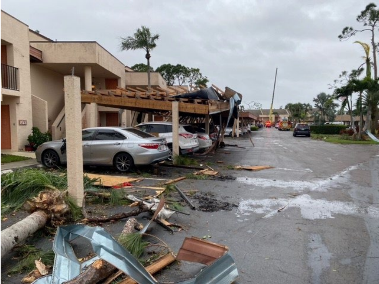
Figure 57 Damage in Lee County from an EF1 Tornado
